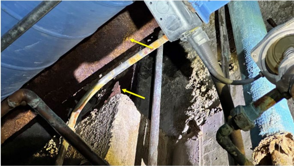
Photograph 1. A steel joists and column at top with corrosion.
